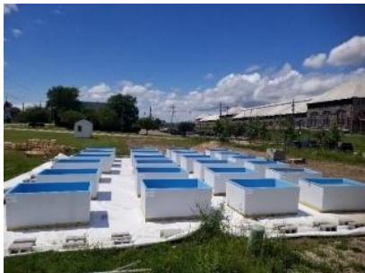
Early stage construction of CFRE’s outdoor mesocosm facility, which will house 24 fiberglass tanks.
